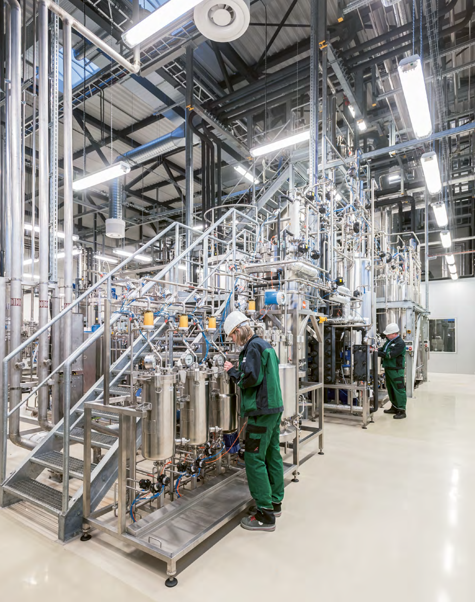
Fermentation plant for the cultivation of various microorganisms (cascade from 10 to 10,000 liters)
