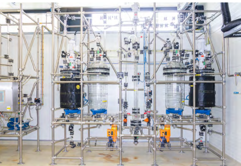
Extraction plant with DN80 countercurrent extraction column
